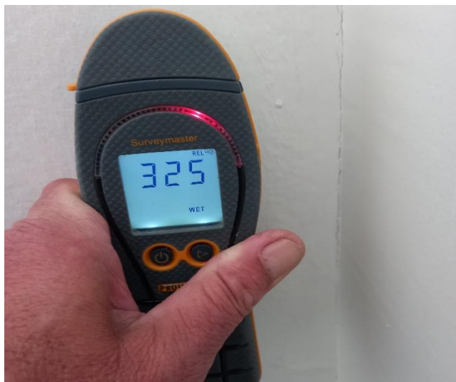
Elevated moisture levels in corner of front bedroom
