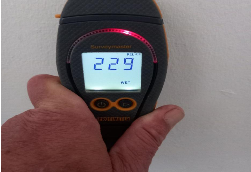
Elevated moisture levels on bedroom wall opposite the bath
