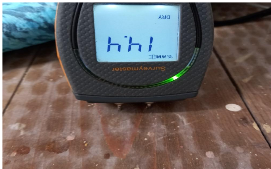
Normal moisture of 14.4% in front bedroom floor
